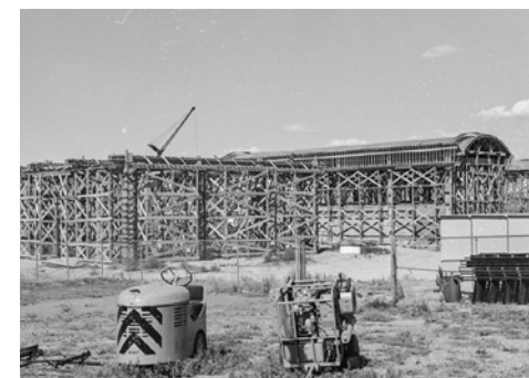
The Armstrong Gym construction rises out of the ground in 1963. (Historical Photo)
